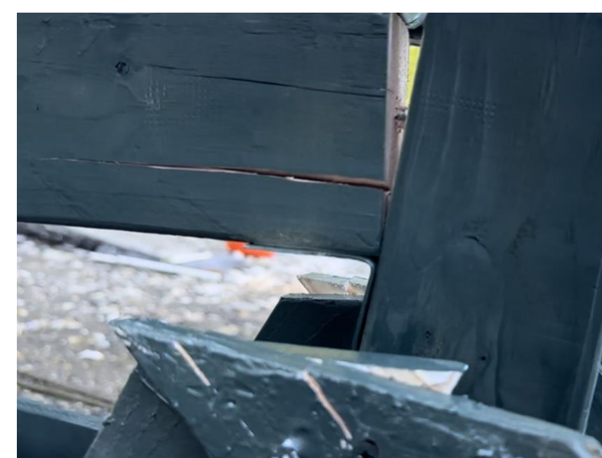
Fig. 5: Point of Failure
